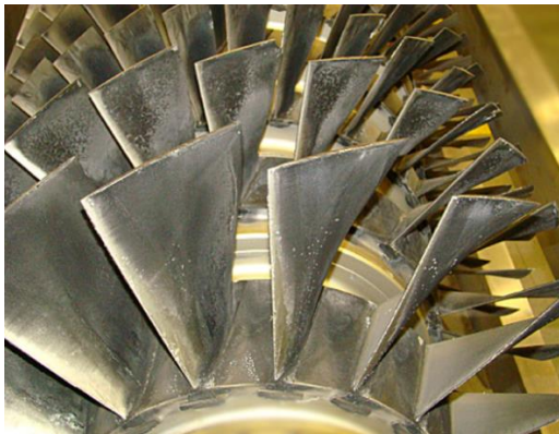
Figure 1. Salt fouling on the compressor blades at 18000 working hours [25]
