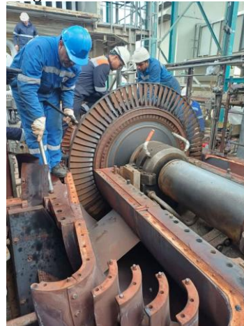
Figure 1. Real View of the Installed Gas Turbine
